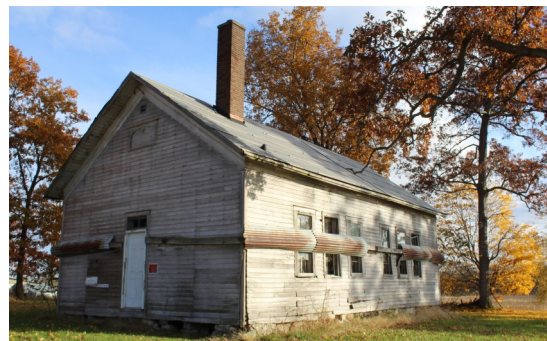
Brownsville #1 School in Cassopolis before repairs by the UGRRSS. The bands will be off!
